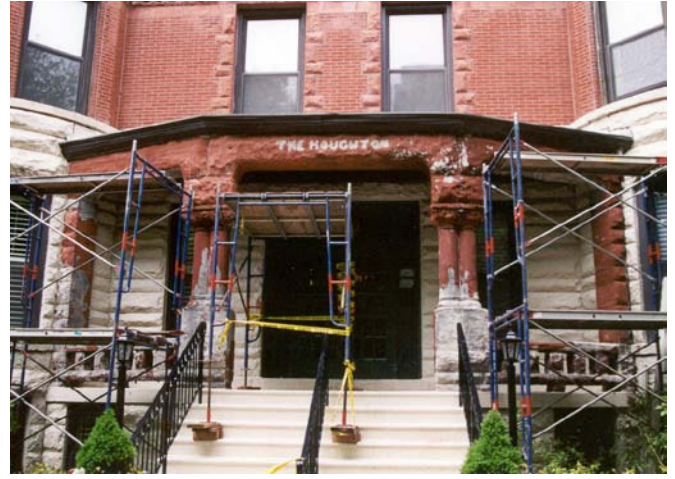
During: Paint has been stripped off of much of the portico.
