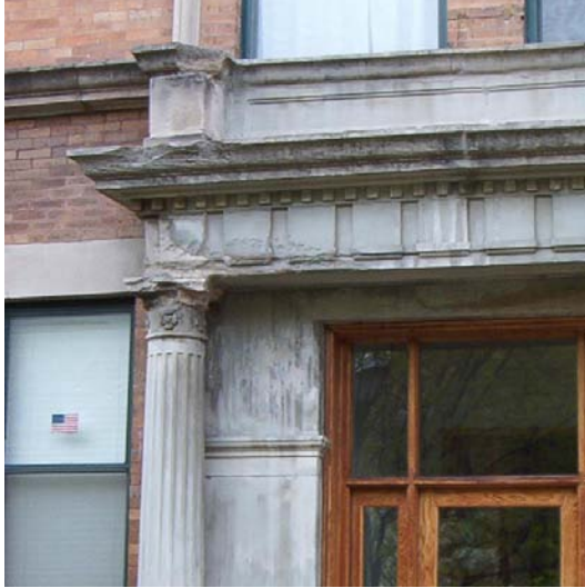
Fig 1. Before. This limestone portico was chemically cleaned to remove stains and discoloration.
