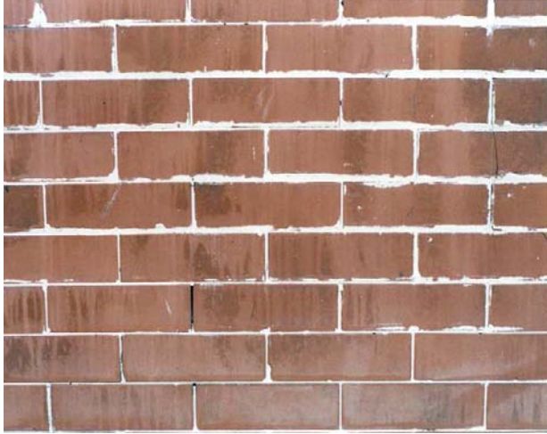
Fig 1. Butter Jointed face brick badly pointed with hard mortar using a high concentration of white portland cement. Originally, it had black mortar, with a flush joint. Mortar was smeared onto the face of the brick, making the joints appear to be thicker than they actually are.
