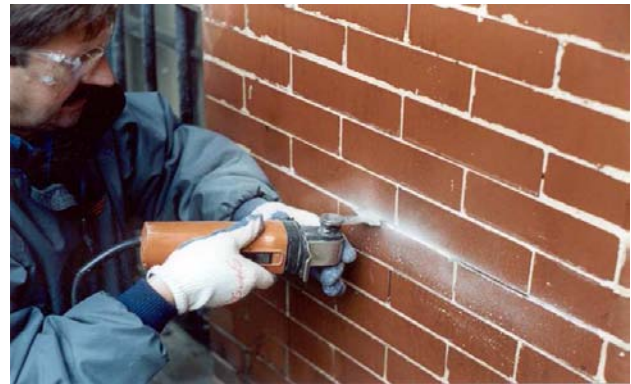
Fig 8. The mortar pictured being removed was particularly hard and the joints were very thin. After attempting to use several different tools, a caulk cutting cutter and a diamond blade proved to work best. When cutting, be careful not to cut too deeply, through all of the mortar. Butter joints were originally laid with mortar only on the edges of the brick.
