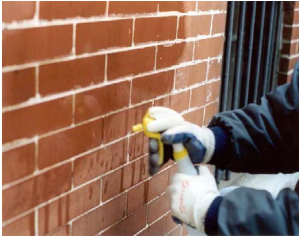
Fig 3. Once the excess mortar has been scraped from the faces of the brick, wet the masonry down with water.
